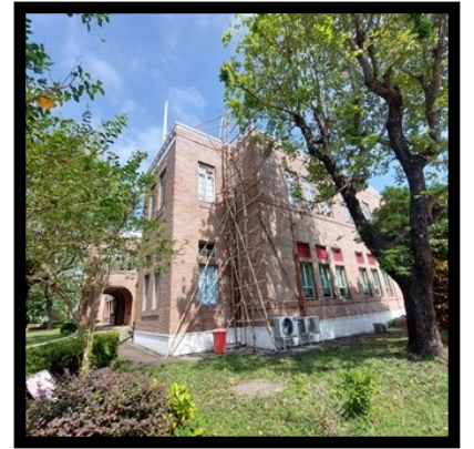
Bamboo scaffolding for a renovation project at the grade 2 listed, Art Deco style HKAC Administration building
